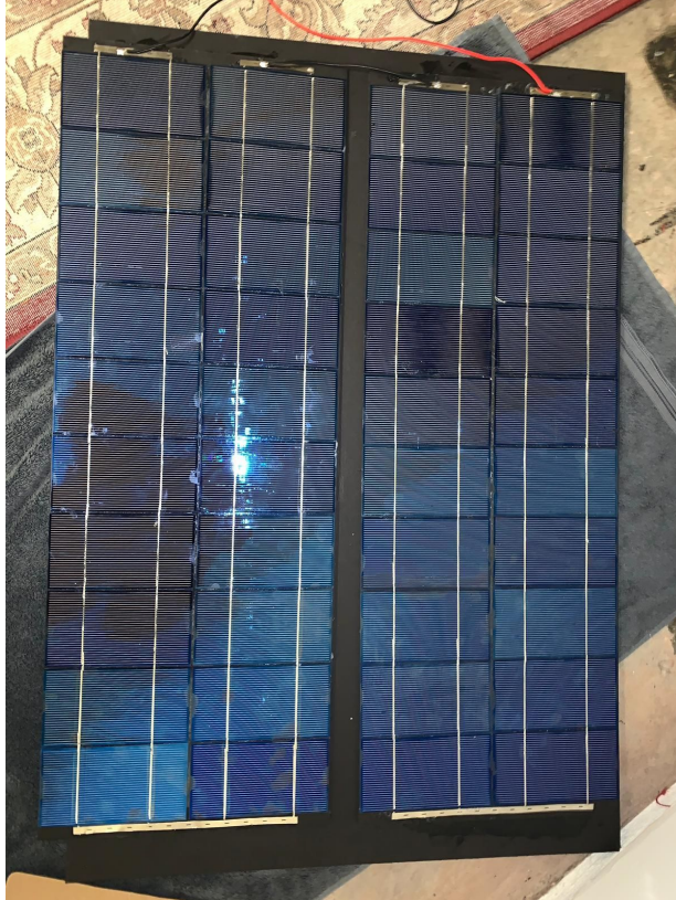
Figure 10: Solar Panel Installed on Platform
